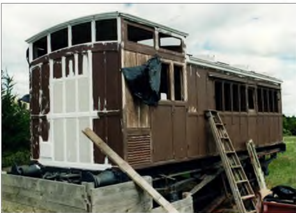
The body was mounted on the painted underframe by a mobile crane. The hole for a wood heater has been filled.
