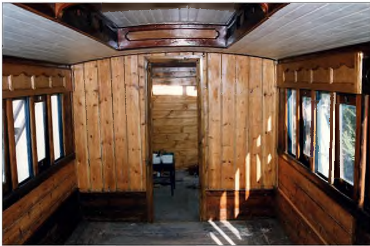
After many months of removing paint the interior was clear varnished with a cream ceiling. Note the windows have also been installed.
